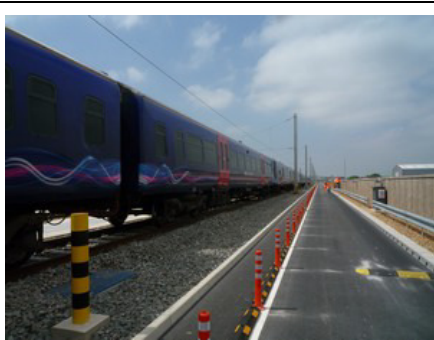
NOISY: sidings for the new train depot. This picture was taken before the new acoustic barrier was put up.
